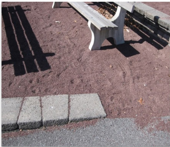
Existing Access Hazard at Band Shell Seating Area
