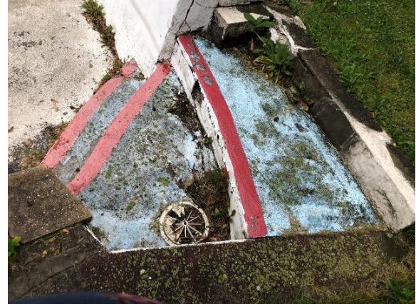
Non-complaint decaying access
