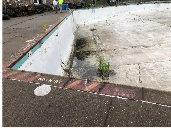
Decayed deep end and apparent water table
