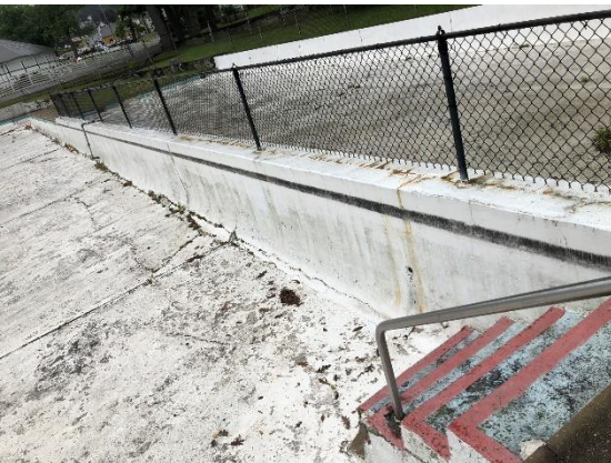
Non-compliant demising wall at Main & Tot Pool
