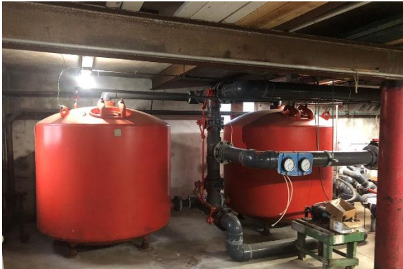
Carbon steel high rate sand filter vessels (4 total)
