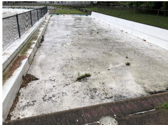
Tot Pool decay with inadequate deck area
