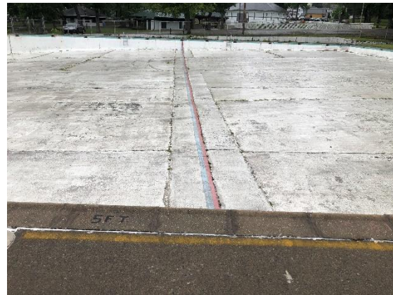
Control joint failure and multiple joints in decay
