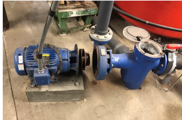
Recirculation pumps & fiberglass hair & lint strainers (2 ea.)
